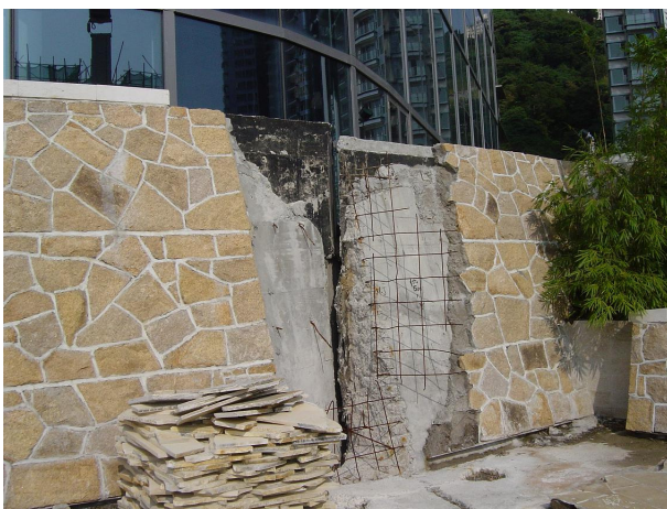
Settlements Induced Cracks
