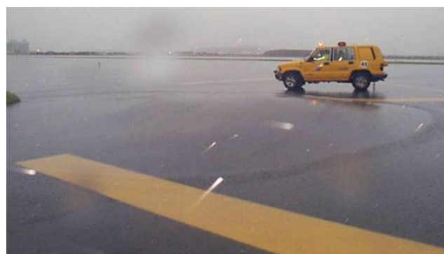
Asphalt dome on taxiway
